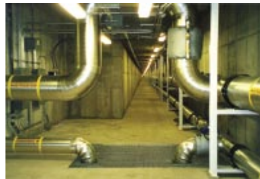
Steam and Utility Tunnel
